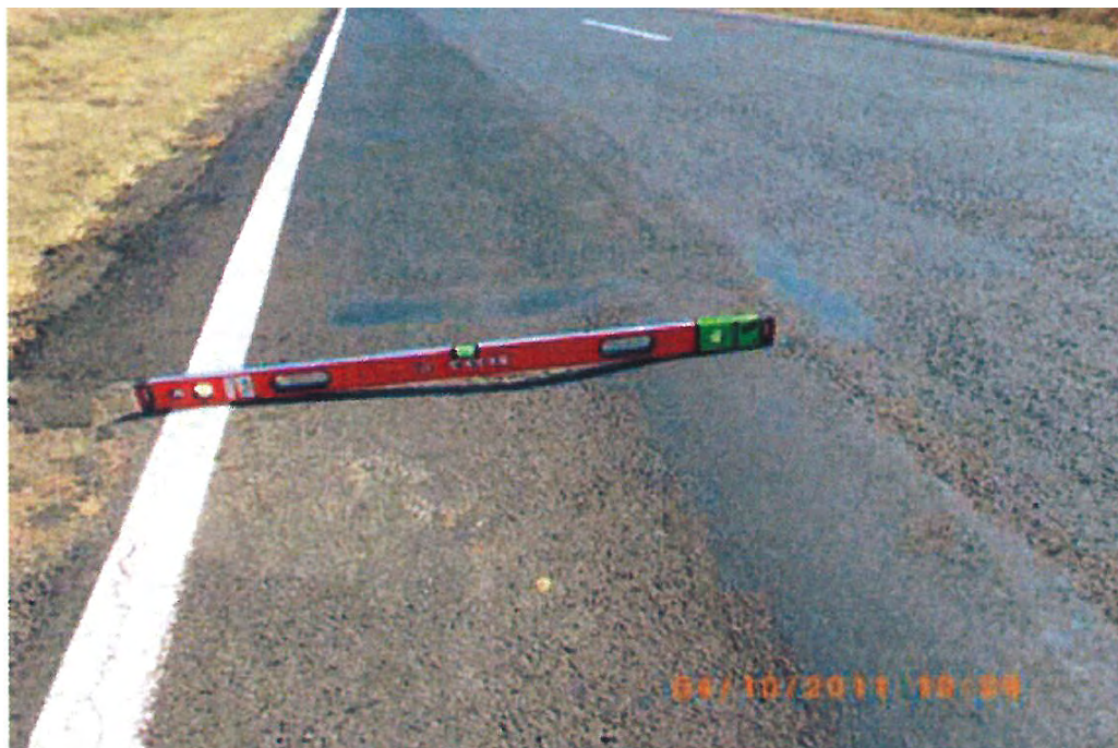
Photo No. 18 - CH 86.51km. Pavement rutting
