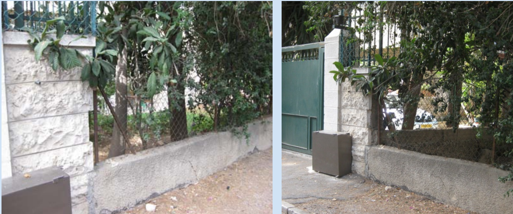
Damaged chain link perimeter fence (right side to centre) abutting the neighbouring stone and palisade fence (left side). ANAO, June 2010.
