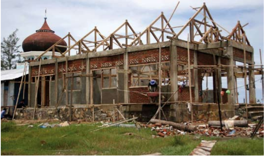
Construction of the new village hall at Kajhu Village, Aceh Besar, under the Aceh Community Infrastructure Program (agreed by Joint Commission Ministers in September 2005). This hall is the first of up to 200 village halls to be rebuilt in the province with technical support and funding from the AIPRD. Photo: AusAID
