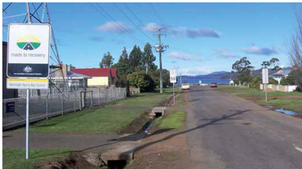
Glamorgan Spring Bay Council, Tasmania: Project No.27: Melbourne Street, Esplanade to Vicary Street, Triabunna—Failed pavement, open gutters. Stormwater drainage construction ($20,000). Photo taken 7 July 2005. Work commenced August 2005.
