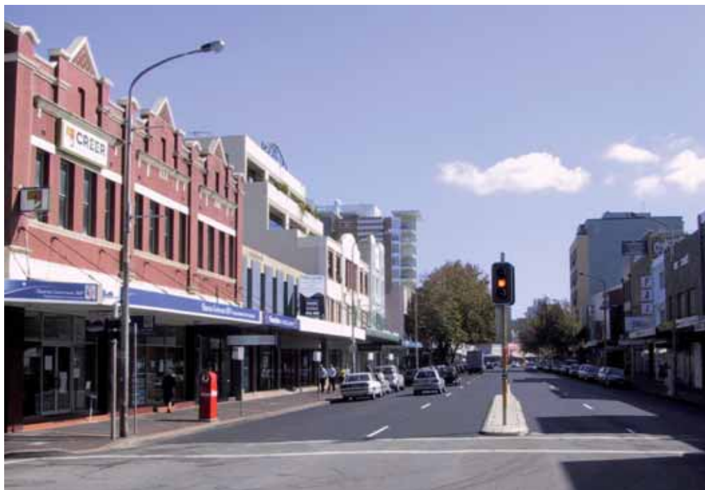
Newcastle City Council, New South Wales: Project No.21: Hunter St Newcastle, Auckland St to Union St—Reconstruction of failed sections of concrete road pavement and resurfacing ($169,000). Photo taken 14 April 2005.
