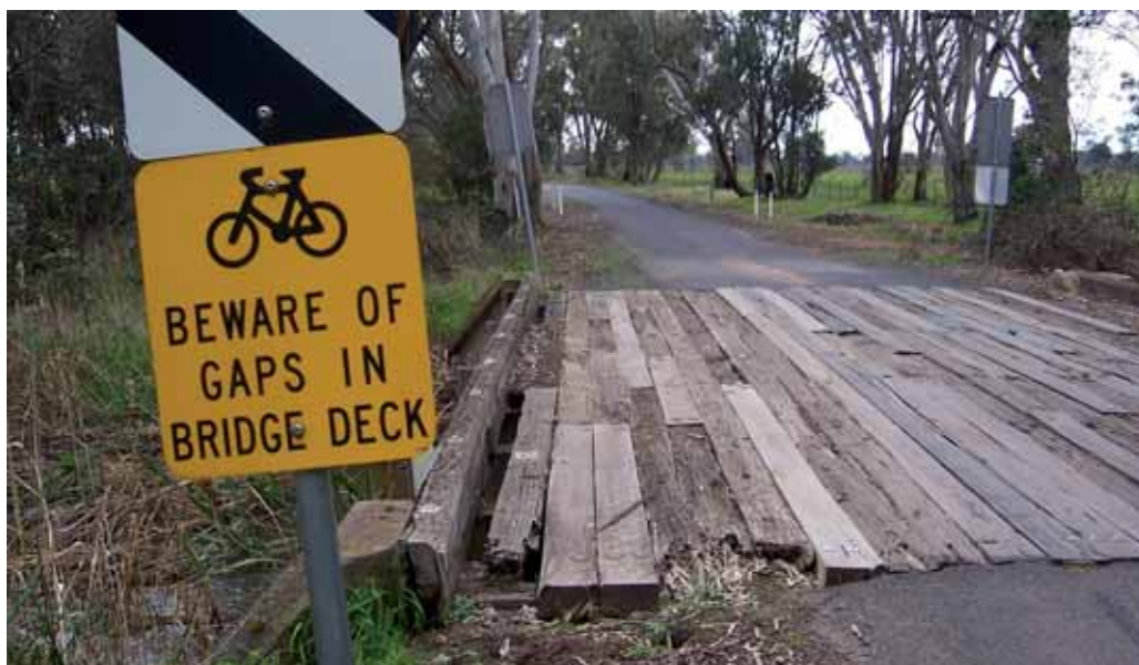
Strathbogrie Shire Council, Victoria, Project No.58: Longwood-Pranjip Road, Pranjip (chainage 6160m): replace existing timber bridge to allow heavy vehicle access ($64,000). Photo taken 18 August 2005.
