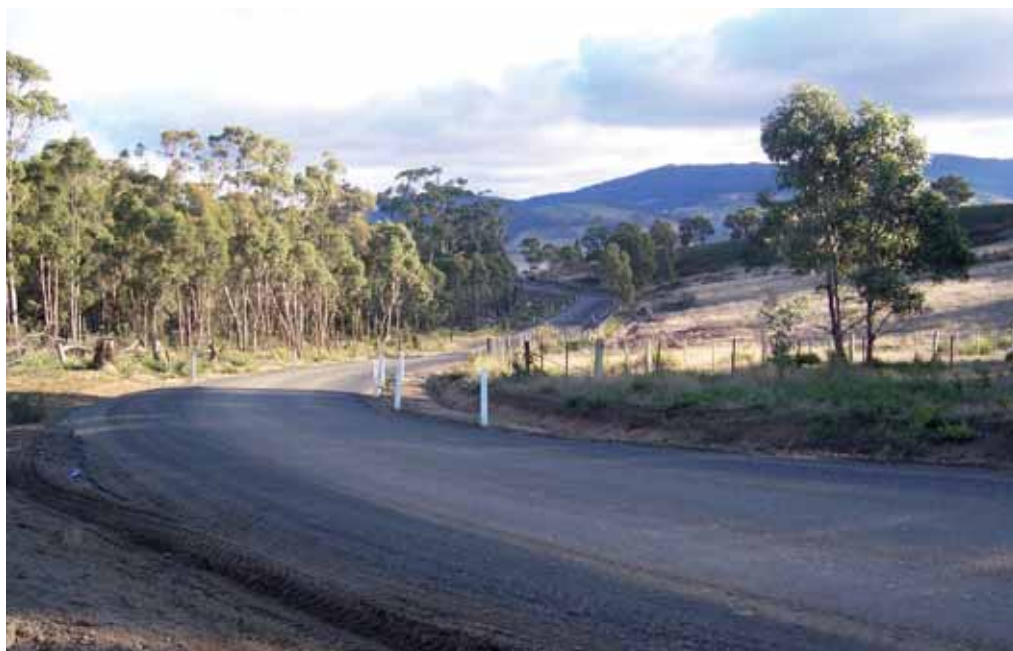
Southern Midlands Council, Tasmania, Project No.53: Eldon Road Colebrook: construct and seal 1.65 kilometres ($80,000). Photo taken 7 July 2005.
