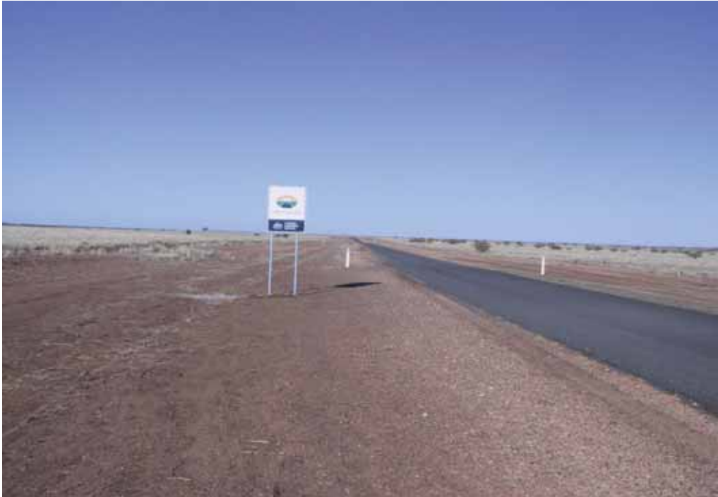
Tambo Shire Council, Queensland, Project No.7: Mt Playfair Road: bitumen sealing for 9 kilometres ($167,000). Photo taken 2 June 2005.
