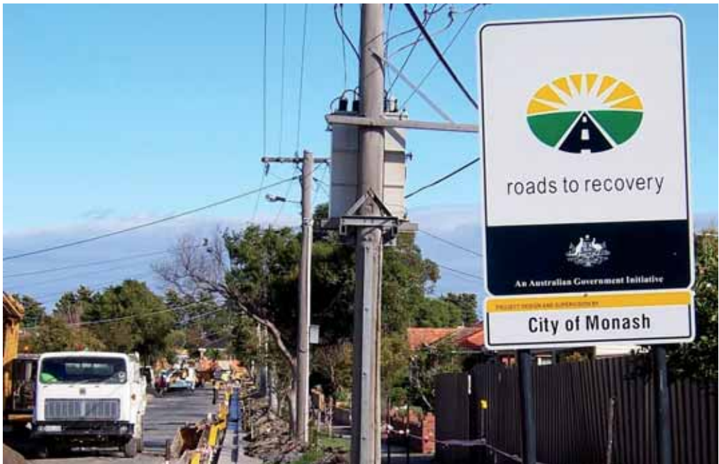
Monash City Council, Victoria, Project No.8: Dermot Street between Delia Street and Devoy Street, Oakleigh South: refurbishment of road ($238,287). Photo taken 10 May 2005 when work was in progress.
