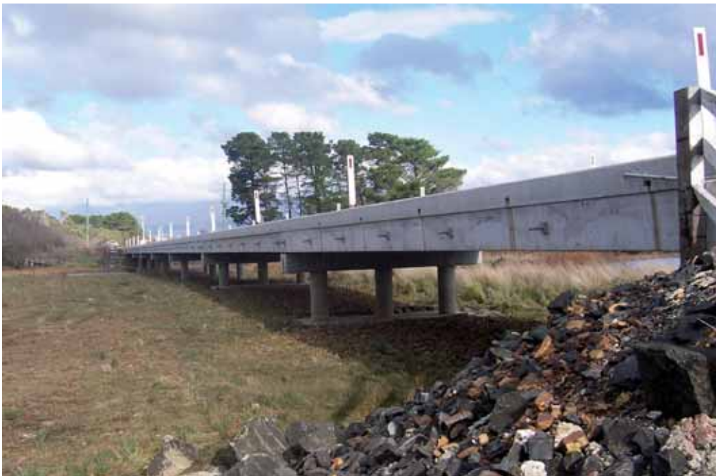
Northern Midlands Council, Tasmania, Project No.6: replacement of Stewarton Bridge No.1965 located on Barton Road ($575,874). Photo taken 6 July 2005.
